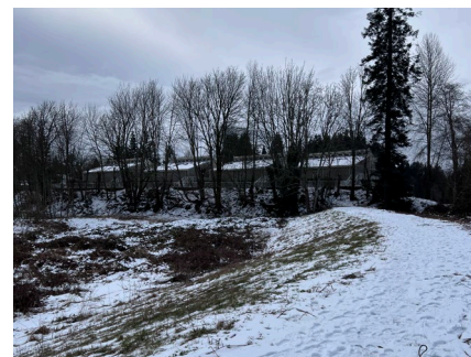
Figure 6-16: Condensory Dike, looking upstream with Puntledge River on the right. (Credit: Ebbwater, 27 Feb 2023).
