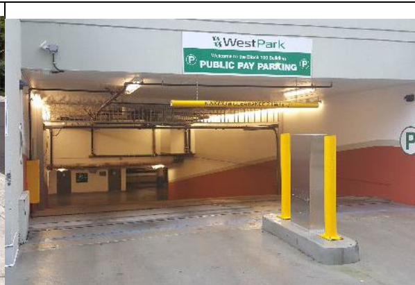
FloodBreak barrier (not activated) at Block 100, Vancouver. (Credit: FloodBreak).
